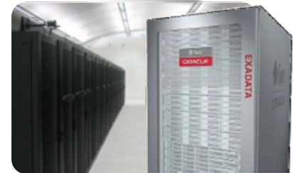
Enterprise Data Center
